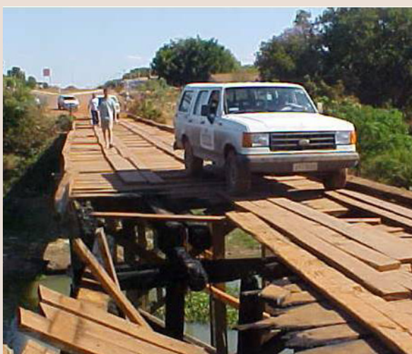
Corruption leads to misappropriation of municipal funds. Pictured above: an unsafe vehicle purchased for use as a school bus and a poorly constructed bridge.
