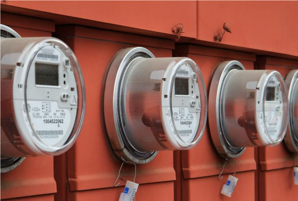
Electricity meters track residential energy use. Photo: Shutterstock.com
