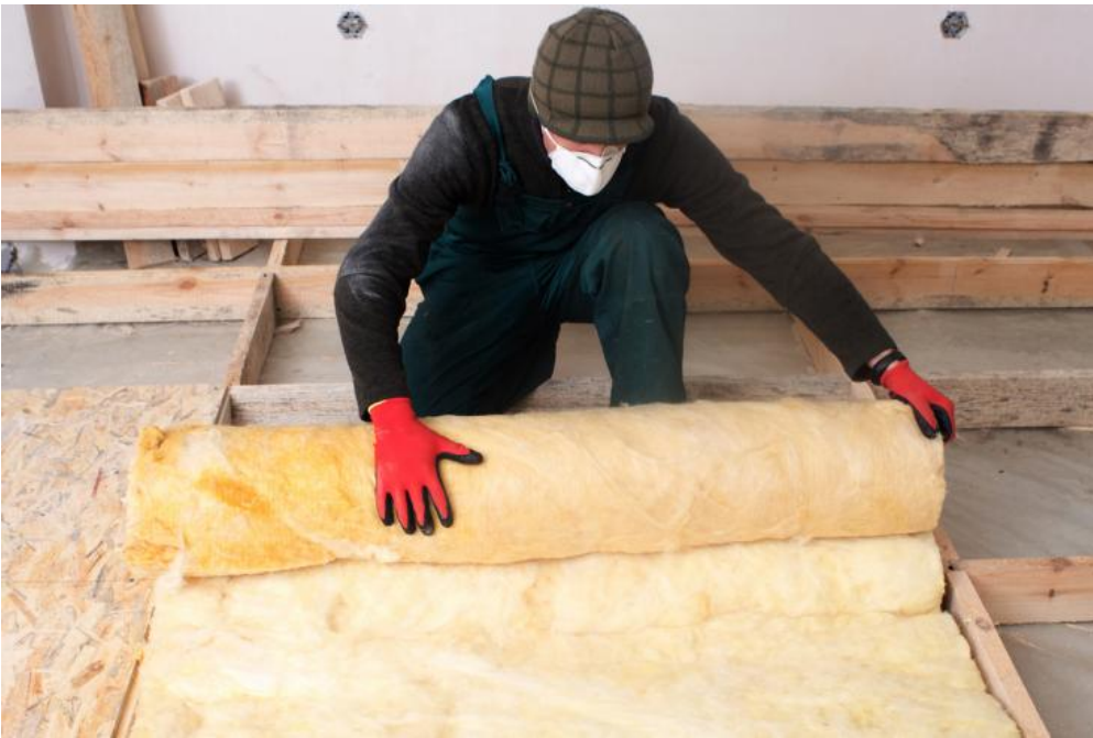
Home floor insulation. Photo: Shutterstock.com
