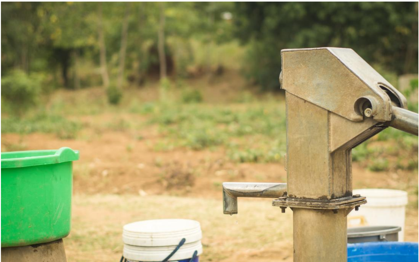
A water point in Malawi.
