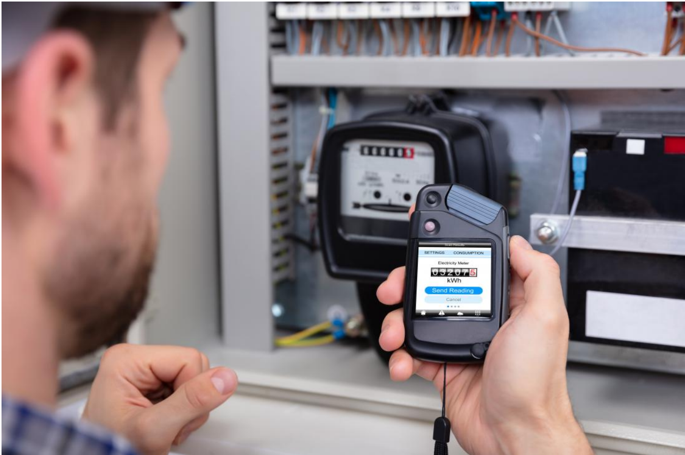
A technician reads a meter.
