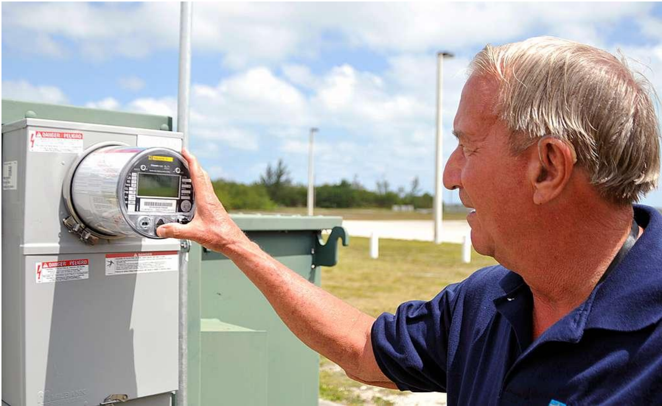
Man performs a check on a smart meter.
